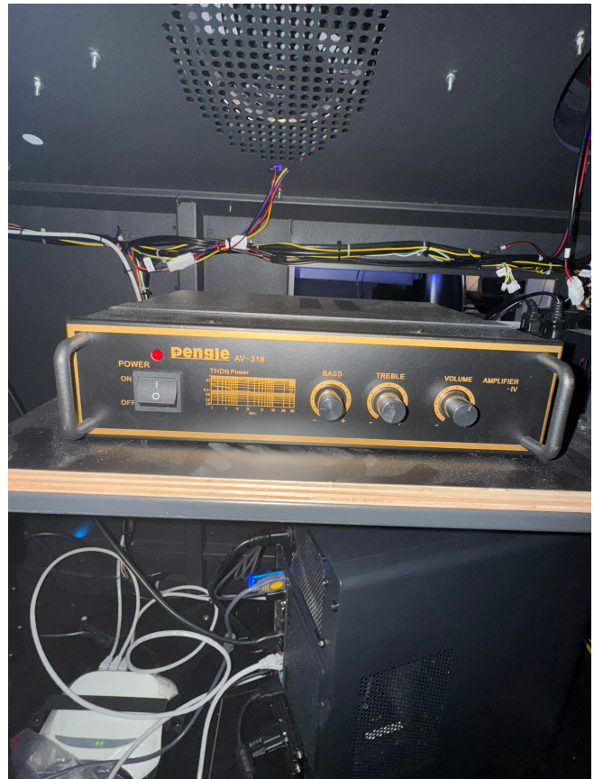
Figure 11: Amplifier powered on
